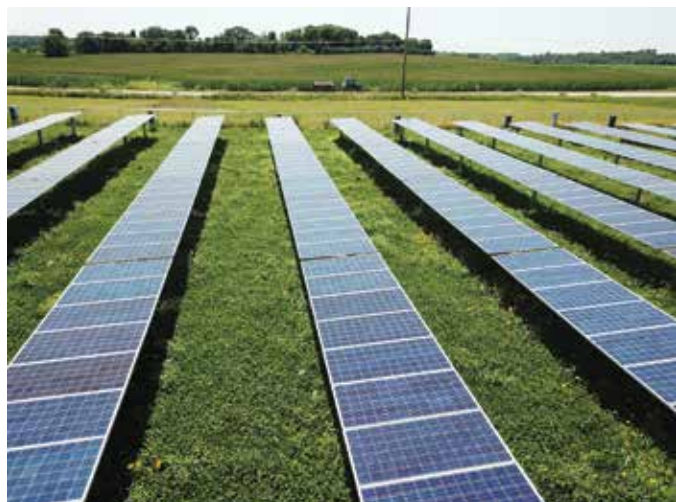
The Transition Energy Solar Project in Richland Electric Cooperative's service territory has 396 photovoltaic tracker panels.
